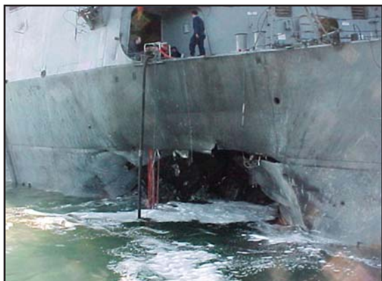
A huge explosion blew a hole in the hull of the USS Cole, a Navy destroyer, as she was moored at Aden port to refuel.
